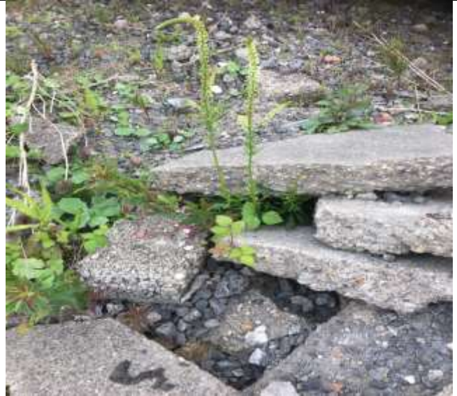
Photo 2: A pile of broken concrete and artificial cobbles/gravel supporting ruderal colonisers (eg. weld and rosebay willowherb). This brownfield habitat type is a localised feature of the Survey Area, particularly in the south-eastern part of the Survey Area near the car park
